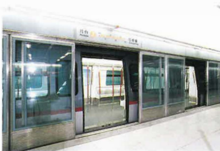
Platform screen doors. 月台幕門
